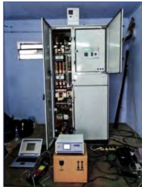
Power Quality Measurement in progress
